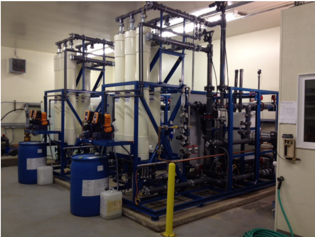
Water Plant Membrane Skids
