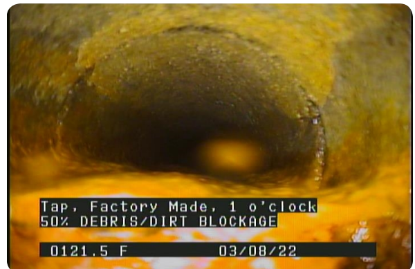
Tap, Factory Made at 121.5 feet, 1 o'clock, 4 in | 50% DEBRIS/DIRT BLOCKAGE
