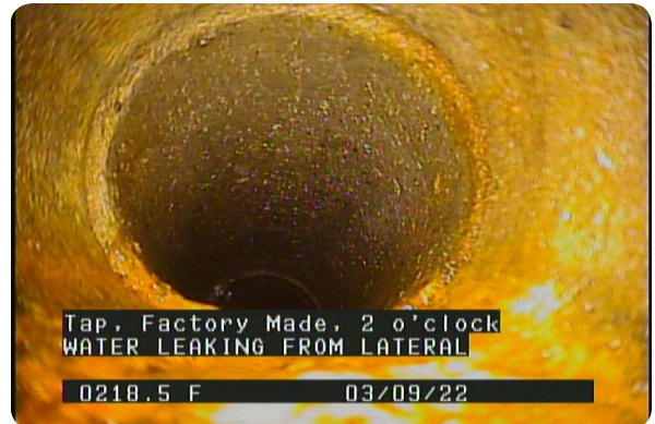
Tap, Factory Made at 218.5 feet, 2 o'clock, 4 in | WATER LEAKING FROM LATERAL
