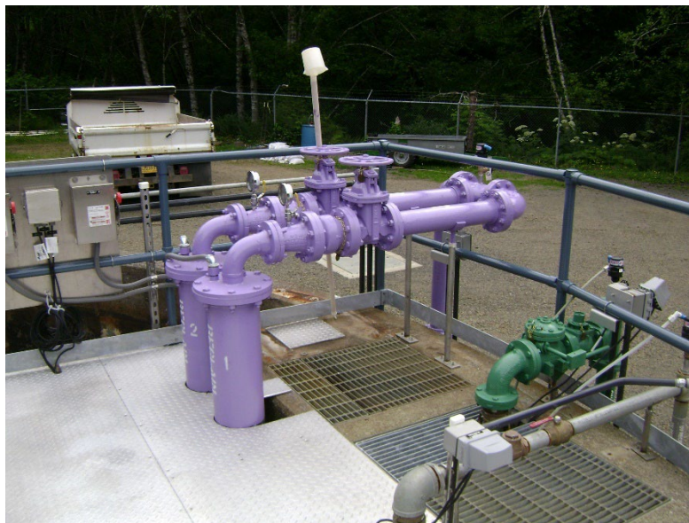
Reclaimed Water Pump Station
