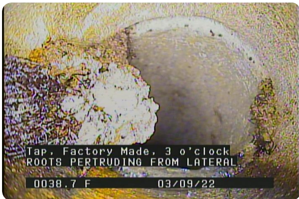
Tap, Factory Made at 038.7 feet, 3 o'clock, 4 in | ROOTS PERTRUDING FROM LATERAL
