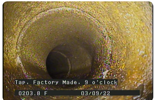
Tap, Factory Made at 203.8 feet, 9 o'clock, 4 in
