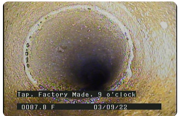
Tap, Factory Made at 087.8 feet, 9 o'clock, 4 in
