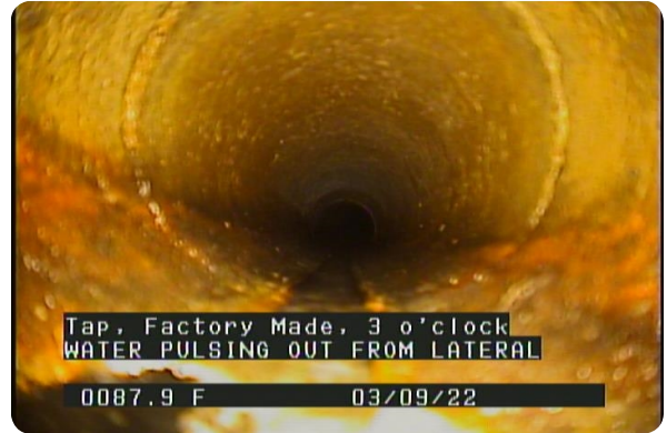
Tap, Factory Made at 087.9 feet, 3 o'clock, 4 in | WATER PULSING OUT FROM LATERAL
