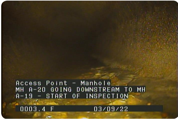
Access Point - Manhole at 000.0 feet | MH A-20 GOING DOWNSTREAM TO MH A-19 - START OF INSPECTION
