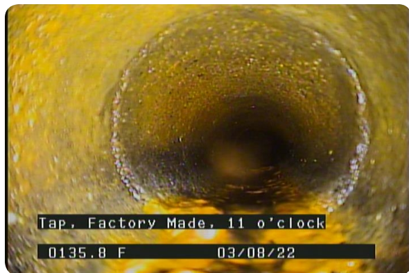
Tap, Factory Made at 135.8 feet, 11 o'clock, 4 in
