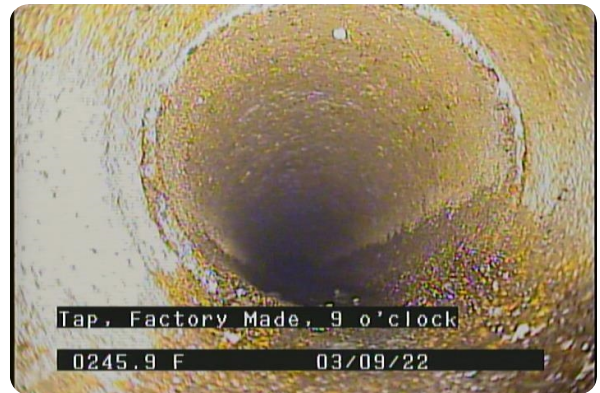
Tap, Factory Made at 245.9 feet, 9 o'clock, 4 in
