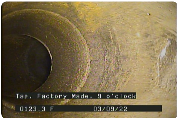
Tap, Factory Made at 123.3 feet, 9 o'clock, 4 in
