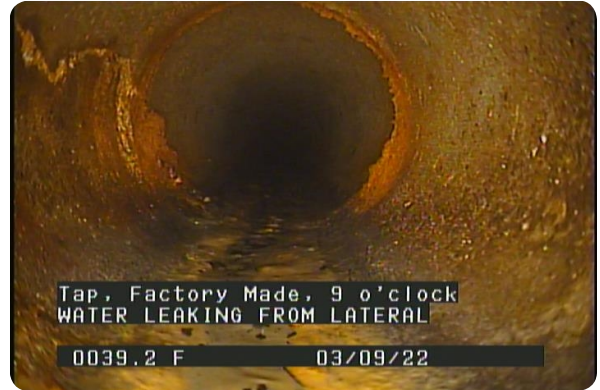
Tap, Factory Made at 039.2 feet, 9 o'clock, 4 in | WATER LEAKING FROM LATERAL
