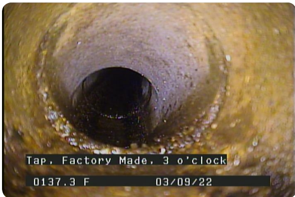
Tap, Factory Made at 137.3 feet, 3 o'clock, 4 in
