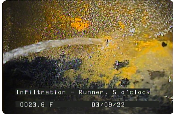
Infiltration - Runner at 023.6 feet, 5 o'clock
