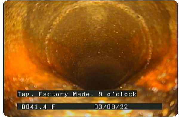
Tap, Factory Made at 041.4 feet, 9 o'clock, 4 in
