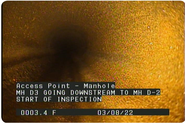
Access Point - Manhole at 000.0 feet | MH D3 GOING DOWNSTREAM TO MH D-2 START OF INSPECTION
