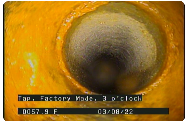
Tap, Factory Made at 057.9 feet, 3 o'clock, 4 in
