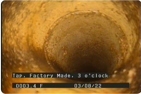
Tap, Factory Made at 003.4 feet, 3 o'clock, 4 in
