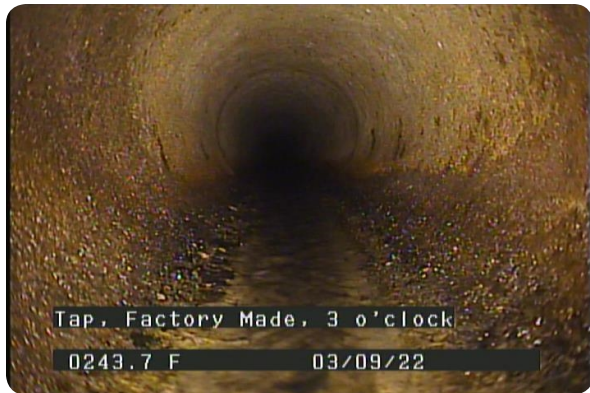
Tap, Factory Made at 243.7 feet, 3 o'clock, 4 in
