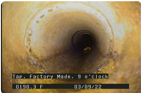
Tap, Factory Made at 190.3 feet, 9 o'clock, 4 in
