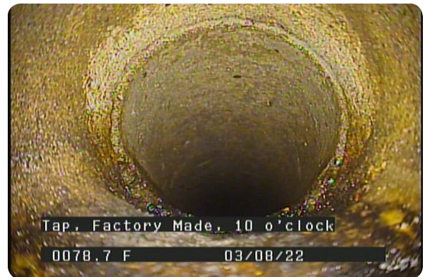
Tap, Factory Made at 078.7 feet, 10 o'clock, 4 in
