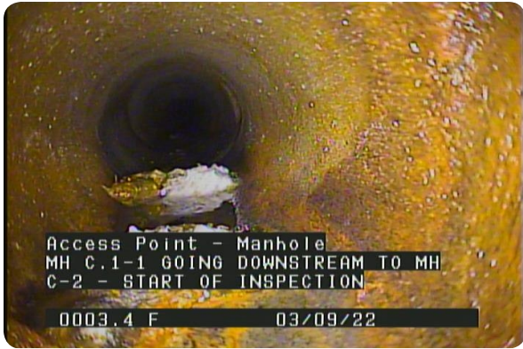
Access Point - Manhole at 000.0 feet | MH C.1-1 GOING DOWNSTREAM TO MH C-2 - START OF INSPECTION
