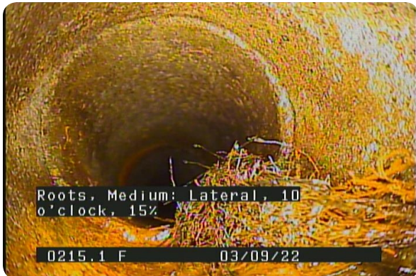
Roots, Medium: Lateral at 215.1 feet, 10 o'clock, 15%
