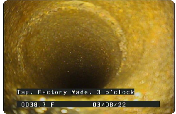
Tap, Factory Made at 038.7 feet, 3 o'clock, 4 in
