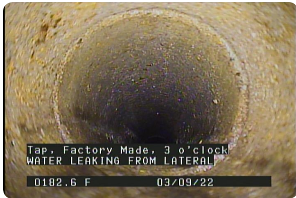
Tap, Factory Made at 182.6 feet, 3 o'clock, 4 in | WATER LEAKING FROM LATERAL
