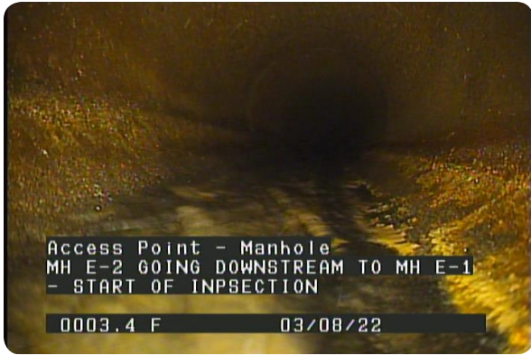
Access Point - Manhole at 000.0 feet | MH E-2 GOING DOWNSTREAM TO MH E-1 - START OF INPSECTION
