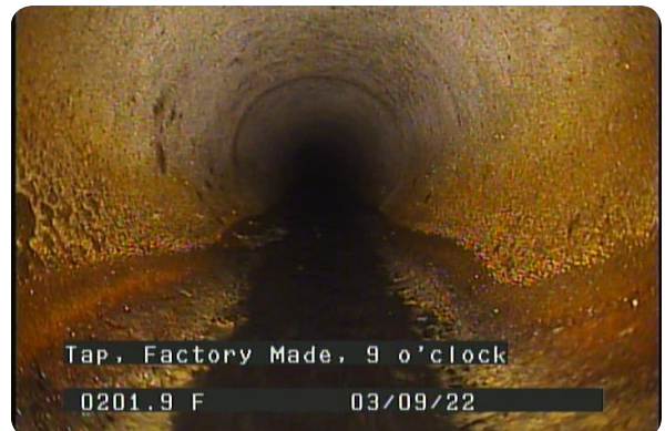
Tap, Factory Made at 201.9 feet, 9 o'clock, 4 in
