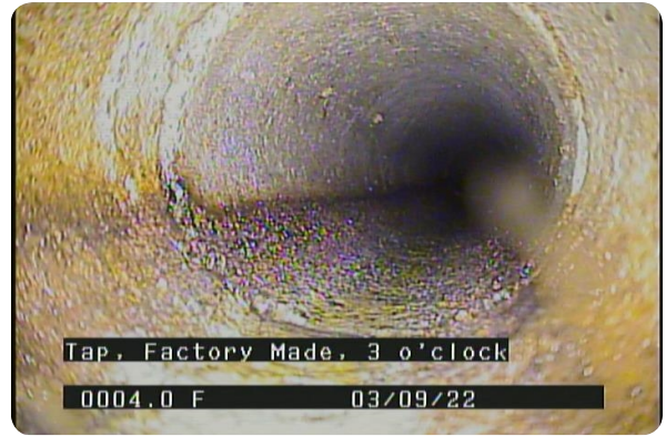
Tap, Factory Made at 003.5 feet, 3 o'clock, 4 in
