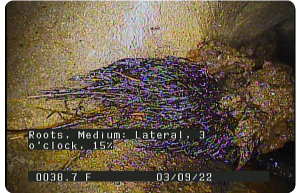
Roots, Medium: Lateral at 038.7 feet, 3 o'clock, 15%
