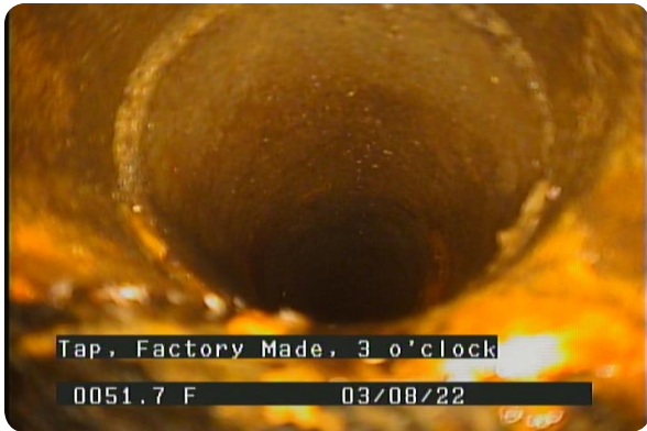
Tap, Factory Made at 051.7 feet, 3 o'clock, 4 in
