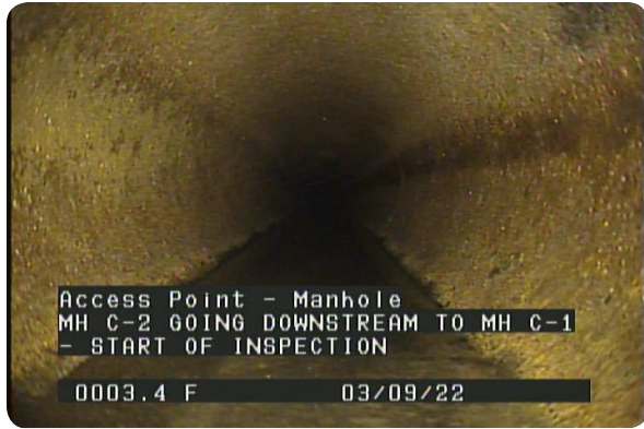
Access Point - Manhole at 000.0 feet | MH C-2 GOING DOWNSTREAM TO MH C-1 - START OF INSPECTION
