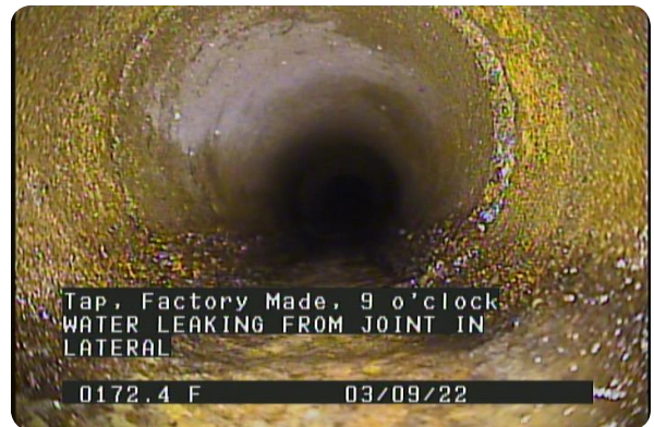
Tap, Factory Made at 172.4 feet, 9 o'clock, 4 in | WATER LEAKING FROM JOINT IN LATERAL
