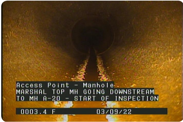
Access Point - Manhole at 000.0 feet | MARSHAL TOP MH GOING DOWNSTREAM TO MH A-20 - START OF INSPECTION
