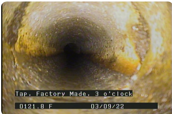
Tap, Factory Made at 121.8 feet, 3 o'clock, 4 in
