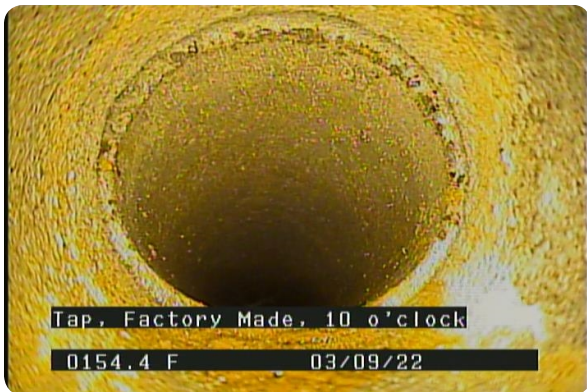
Tap, Factory Made at 154.4 feet, 10 o'clock, 4 in
