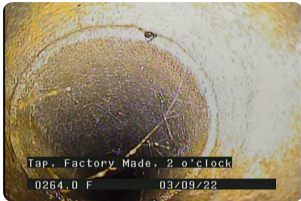
Tap, Factory Made at 264.0 feet, 2 o'clock, 4 in
