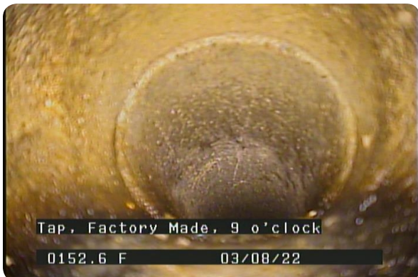
Tap, Factory Made at 152.6 feet, 9 o'clock, 4 in
