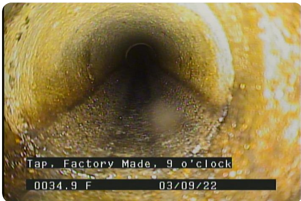
Tap, Factory Made at 034.9 feet, 9 o'clock, 4 in
