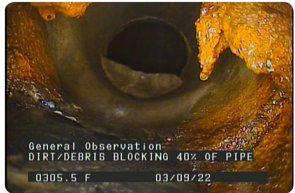
General Observation at 305.5 feet | DIRT/DEBRIS BLOCKING 40% OF PIPE
