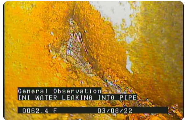
General Observation at 062.4 feet | INI WATER LEAKING INTO PIPE
