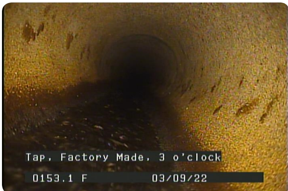
Tap, Factory Made at 153.1 feet, 3 o'clock, 4 in
