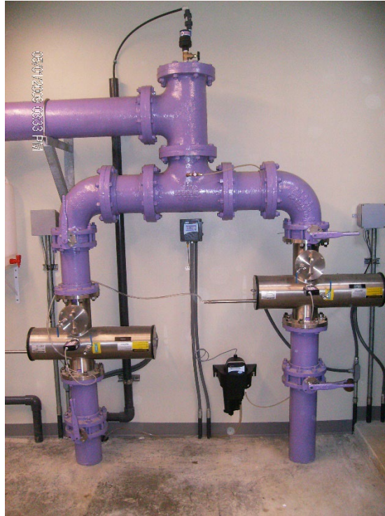
UV Disinfection System
