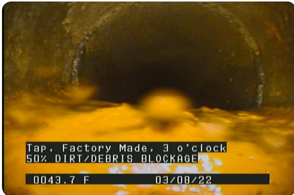
Tap, Factory Made at 043.7 feet, 3 o'clock, 4 in | 50% DIRT/DEBRIS BLOCKAGE
