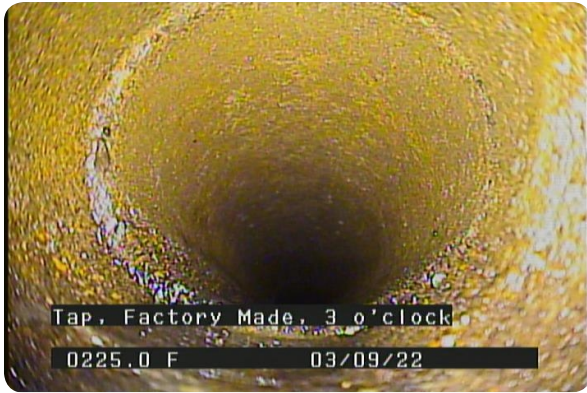
Tap, Factory Made at 225.0 feet, 3 o'clock, 4 in
