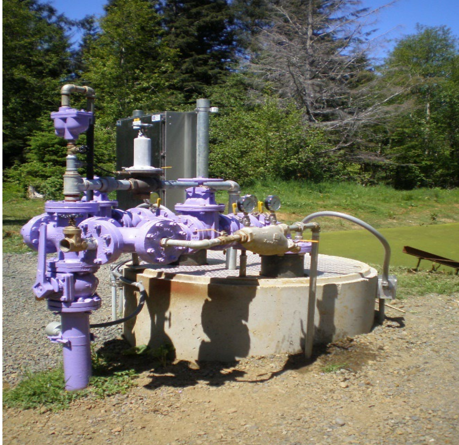
Irrigation Pump Station
