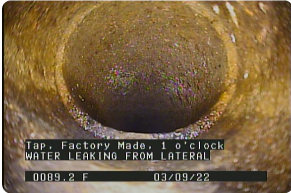
Tap, Factory Made at 089.2 feet, 1 o'clock, 4 in | WATER LEAKING FROM LATERAL
