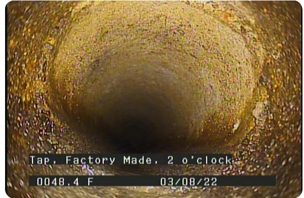
Tap, Factory Made at 048.4 feet, 2 o'clock, 4 in
