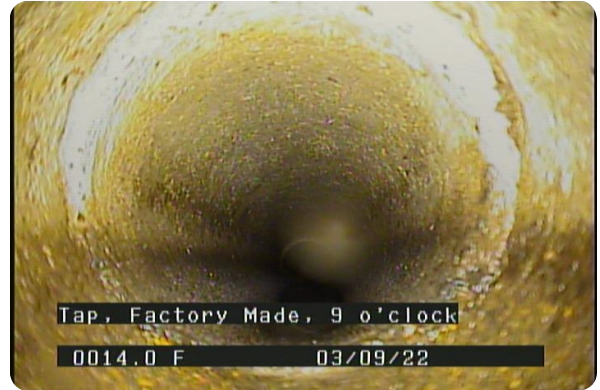
Tap, Factory Made at 014.0 feet, 9 o'clock, 4 in
