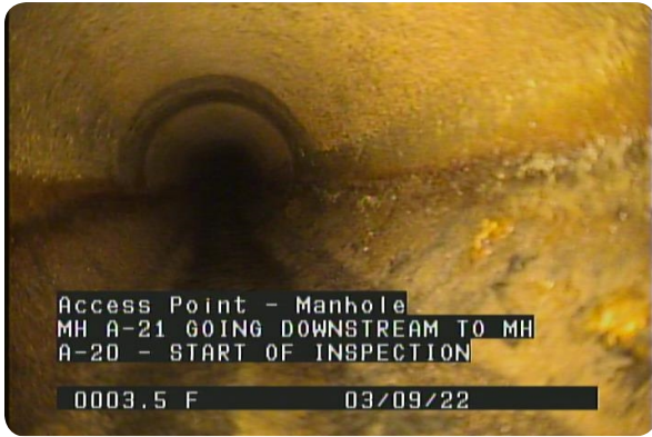
Access Point - Manhole at 000.0 feet | MH A-21 GOING DOWNSTREAM TO MH A-20 - START OF INSPECTION
