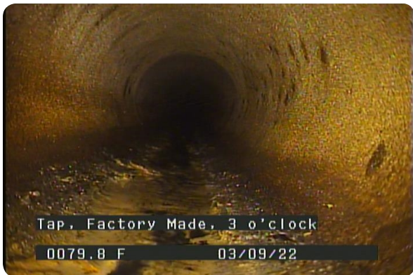
Tap, Factory Made at 079.8 feet, 3 o'clock, 4 in
