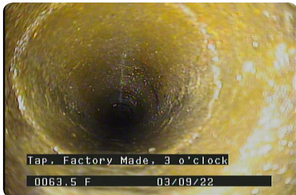
Tap, Factory Made at 057.0 feet, 3 o'clock, 4 in
