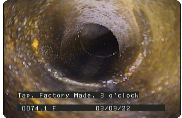
Tap, Factory Made at 074.1 feet, 3 o'clock, 4 in
