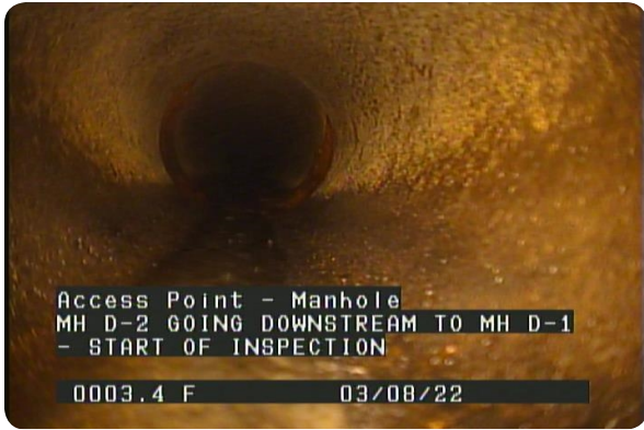
Access Point - Manhole at 000.0 feet | MH D-2 GOING DOWNSTREAM TO MH D-1 - START OF INSPECTION
