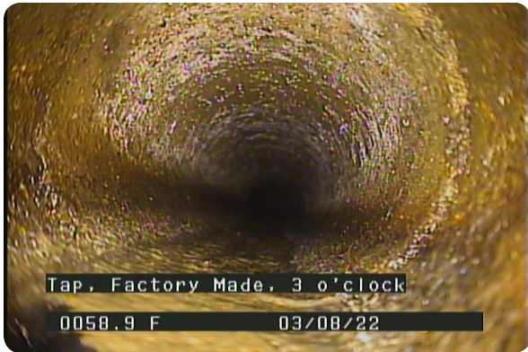
Tap, Factory Made at 058.9 feet, 3 o'clock, 4 in
