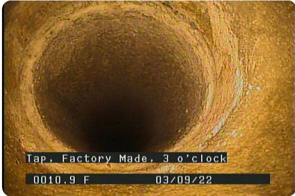
Tap, Factory Made at 010.9 feet, 3 o'clock, 4 in
