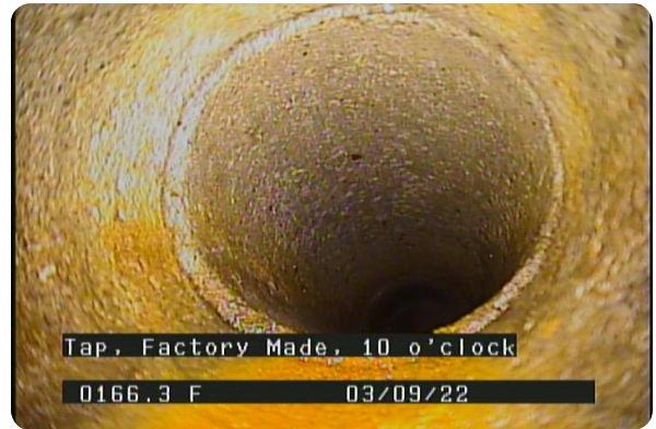
Tap, Factory Made at 166.3 feet, 10 o'clock, 4 in
