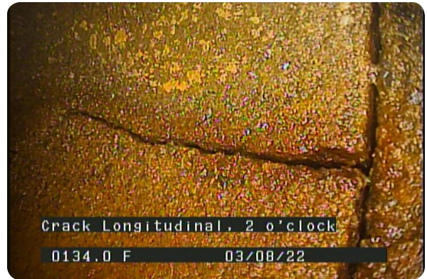
Crack Longitudinal at 134.0 feet, 2 o'clock
