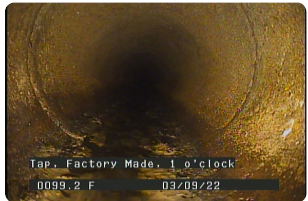
Tap, Factory Made at 099.2 feet, 1 o'clock, 4 in
