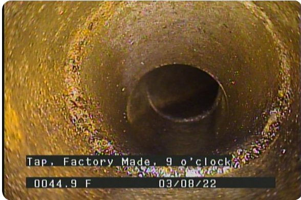
Tap, Factory Made at 044.9 feet, 9 o'clock, 4 in
