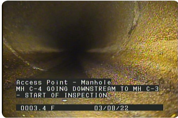
Access Point - Manhole at 000.0 feet | MH C-4 GOING DOWNSTREAM TO MH C-3 - START OF INSPECTION
