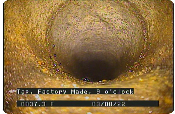
Tap, Factory Made at 037.3 feet, 9 o'clock, 4 in
