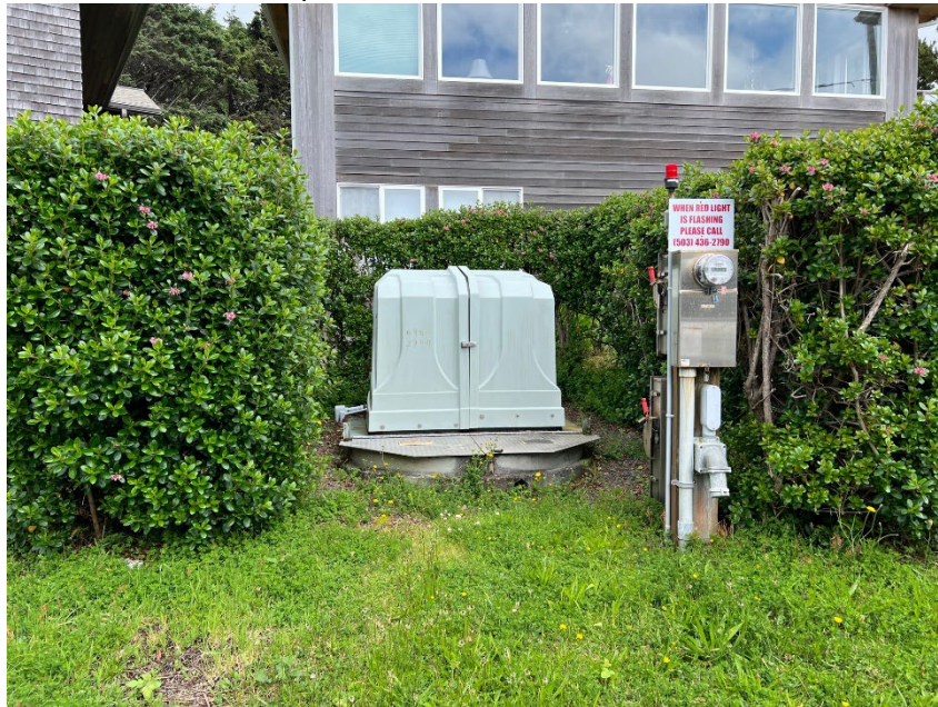
North End Pump Station
