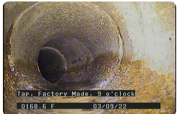
Tap, Factory Made at 168.6 feet, 9 o'clock, 4 in
