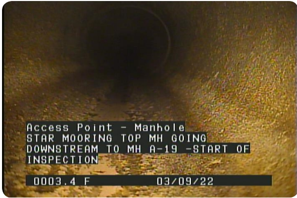
Access Point - Manhole at 000.0 feet | STAR MOORING TOP MH GOING DOWNSTREAM TO MH A-19 -START OF
