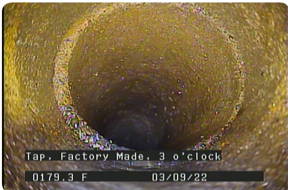
Tap, Factory Made at 179.3 feet, 3 o'clock, 4 in
