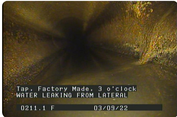
Tap, Factory Made at 211.1 feet, 3 o'clock, 4 in | WATER LEAKING FROM LATERAL
