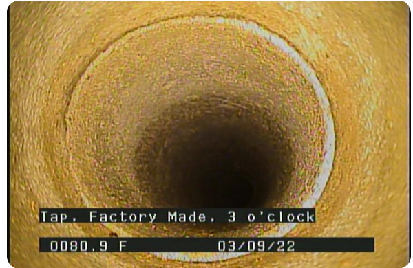
Tap, Factory Made at 080.9 feet, 3 o'clock, 4 in
