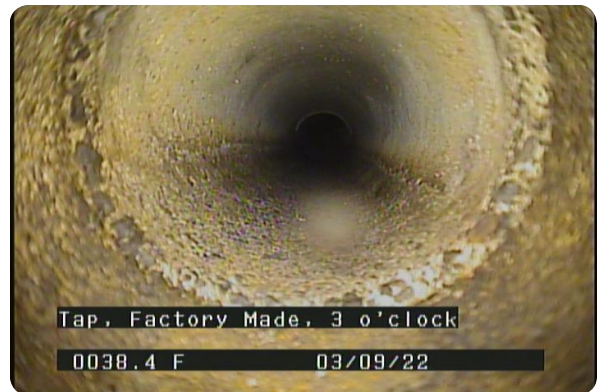
Tap, Factory Made at 038.4 feet, 3 o'clock, 4 in
