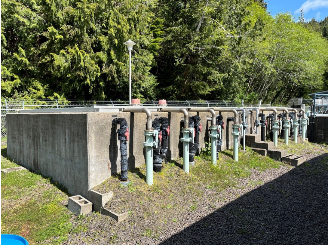
Membrane Filtration System
