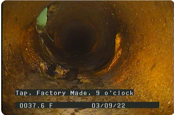
Tap, Factory Made at 037.6 feet, 9 o'clock, 4 in
