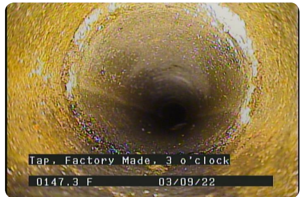
Tap, Factory Made at 147.3 feet, 3 o'clock, 4 in
