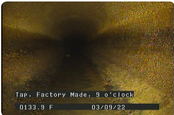
Tap, Factory Made at 133.9 feet, 9 o'clock, 4 in
