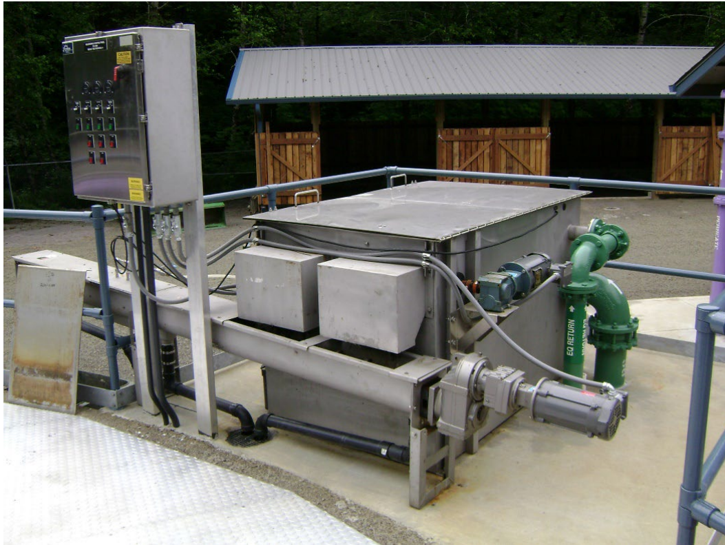
Headworks Raw Screening
