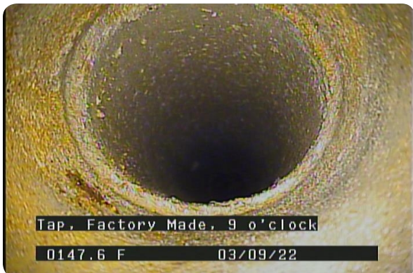
Tap, Factory Made at 147.6 feet, 9 o'clock, 4 in
