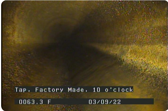
Tap, Factory Made at 063.3 feet, 10 o'clock, 4 in
