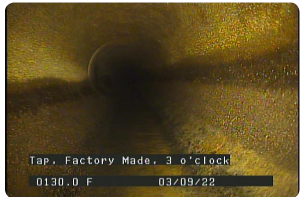
Tap, Factory Made at 130.0 feet, 3 o'clock, 4 in
