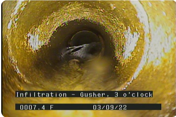
Infiltration - Gusher at 007.4 feet, 3 o'clock
