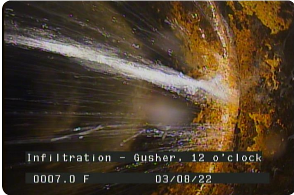
Infiltration - Gusher at 007.0 feet, 12 o'clock
