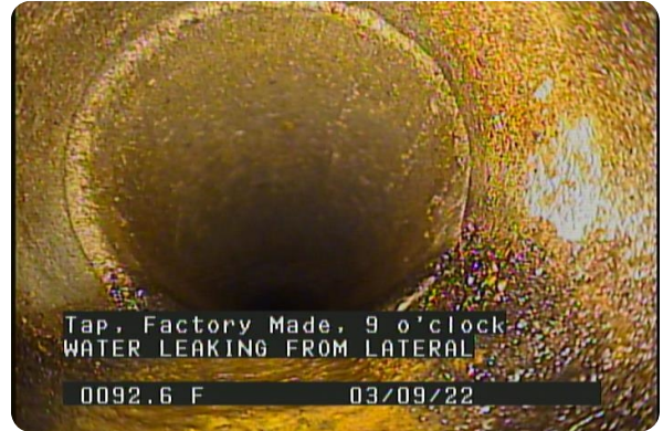
Tap, Factory Made at 092.6 feet, 9 o'clock, 4 in | WATER LEAKING FROM LATERAL
