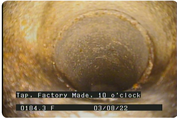
Tap, Factory Made at 184.3 feet, 10 o'clock, 4 in
