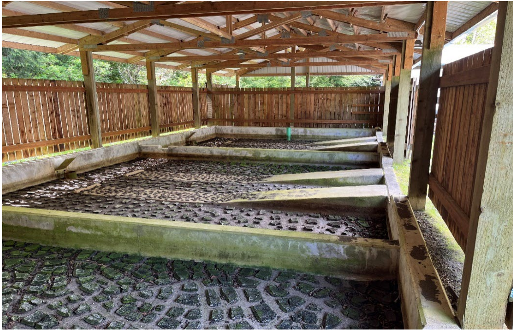
Sludge Drying Beds
