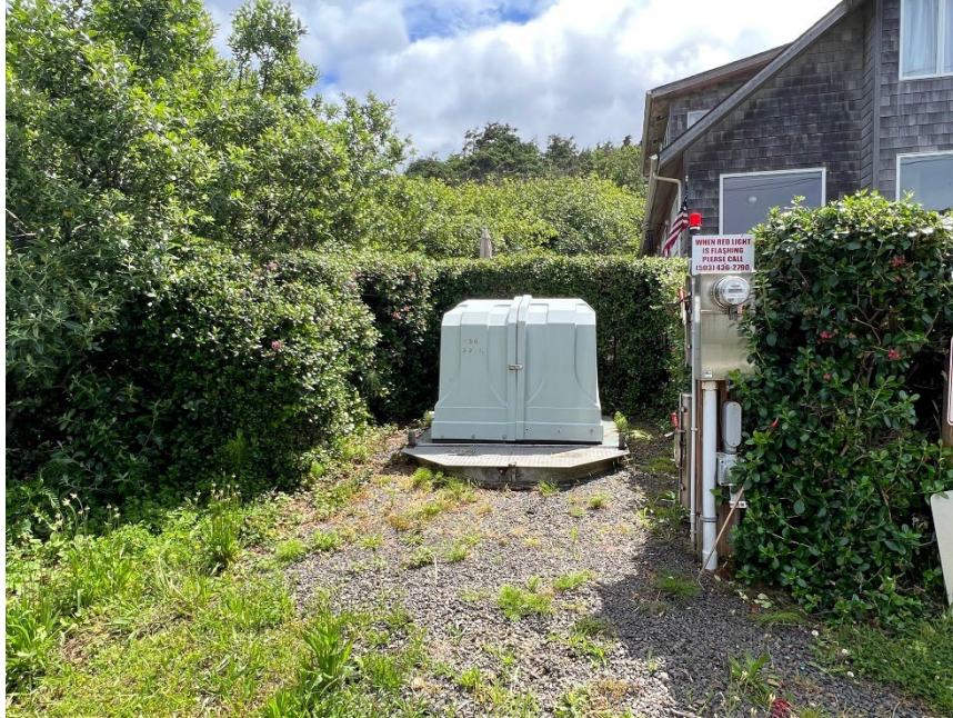
Asbury Pump Station
