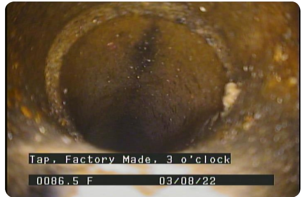
Tap, Factory Made at 086.5 feet, 3 o'clock, 4 in
