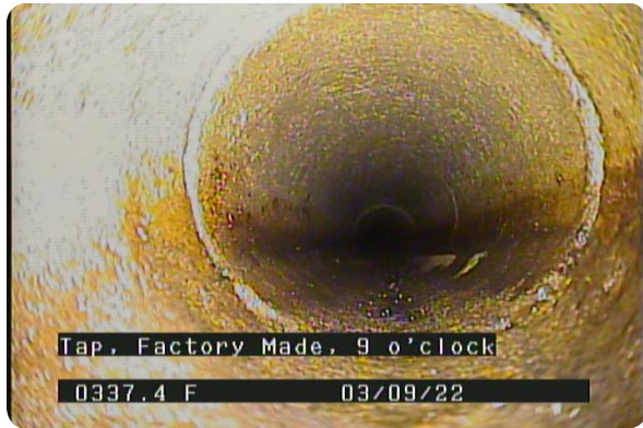
Tap, Factory Made at 337.4 feet, 9 o'clock, 4 in
