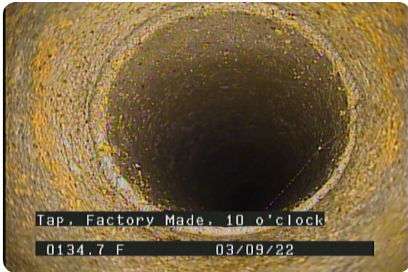
Tap, Factory Made at 134.7 feet, 10 o'clock, 4 in
