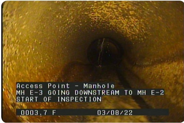
Access Point - Manhole at 000.0 feet | MH E-3 GOING DOWNSTREAM TO MH E-2 START OF INSPECTION
