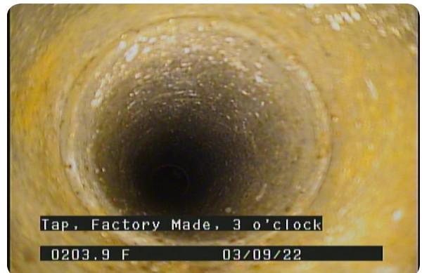
Tap, Factory Made at 203.9 feet, 3 o'clock, 4 in
