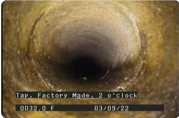
Tap, Factory Made at 032.0 feet, 2 o'clock, 4 in
