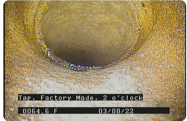
Tap, Factory Made at 064.6 feet, 2 o'clock, 4 in
