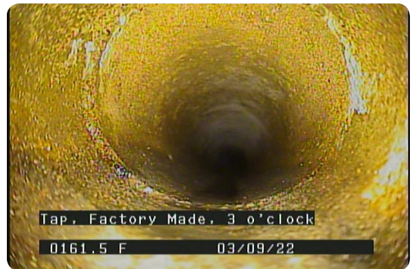
Tap, Factory Made at 161.5 feet, 3 o'clock, 4 in
