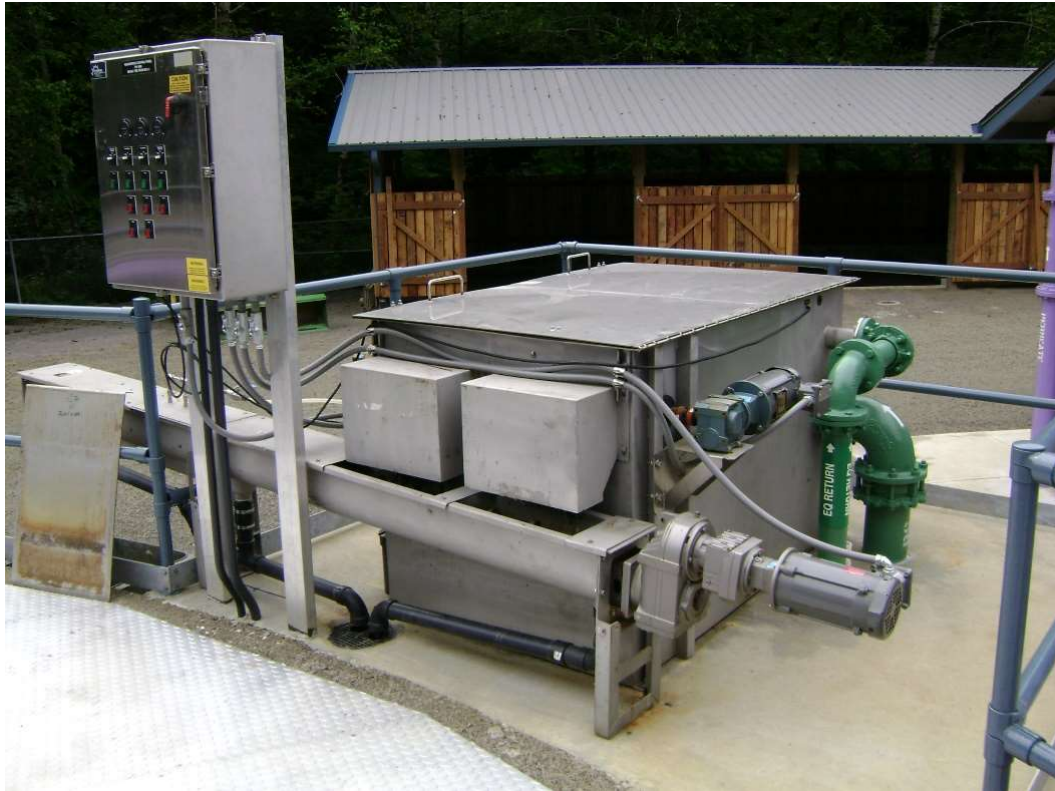
Headworks Raw Screening
