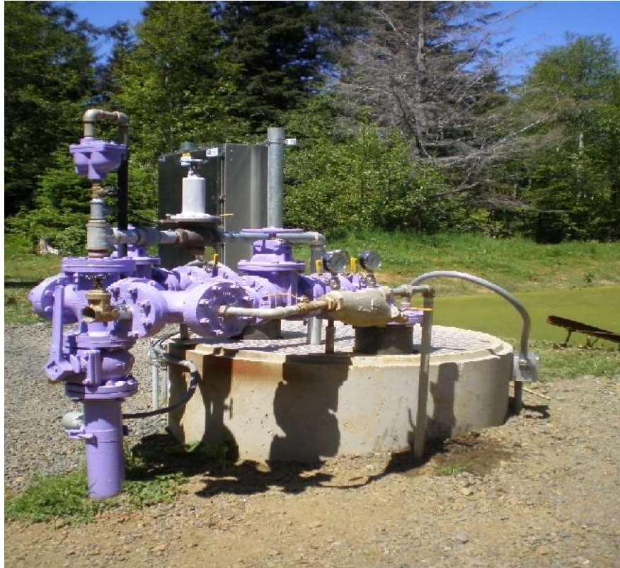
Irrigation Pump Station
