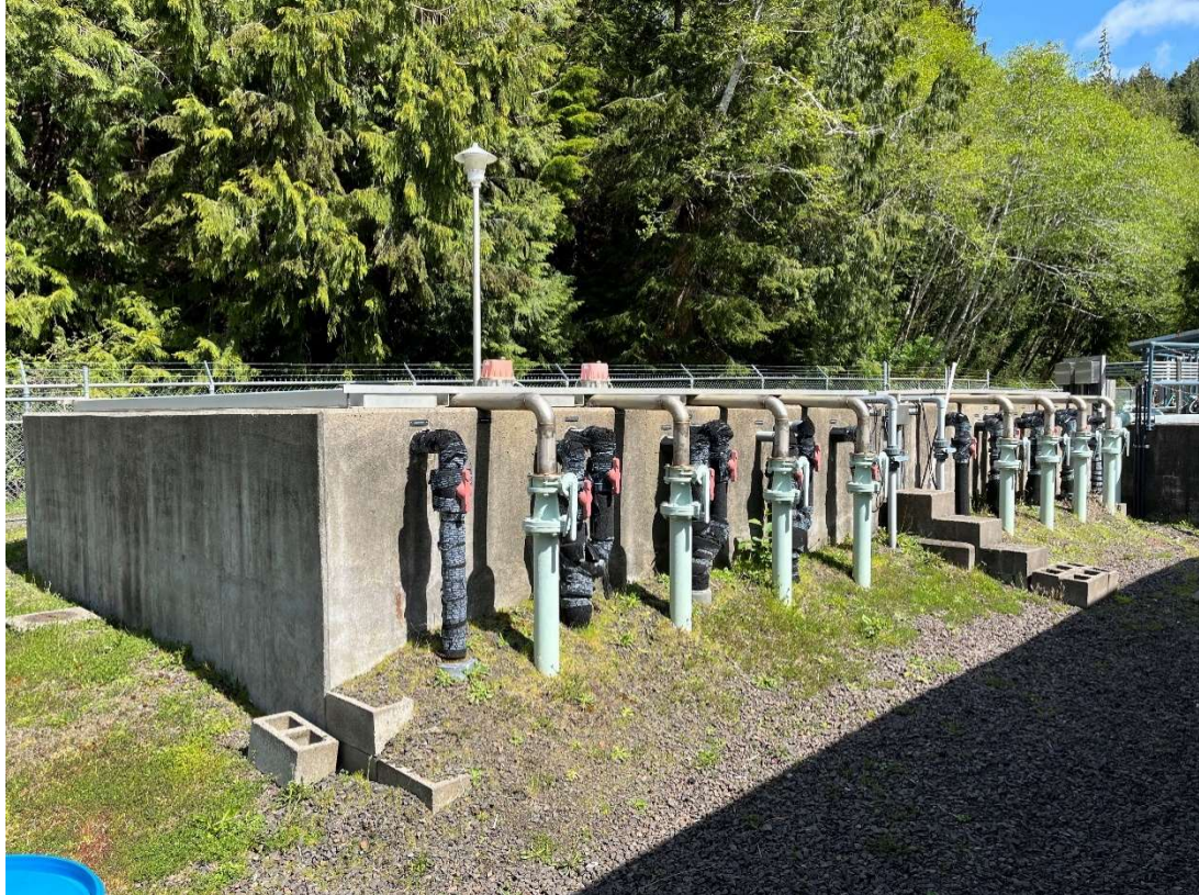
Membrane Filtration System
