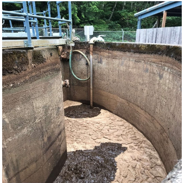
Aerobic Digester No. 2
