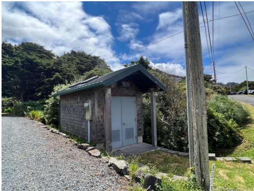
Sally's Alley Pump Station Control building
