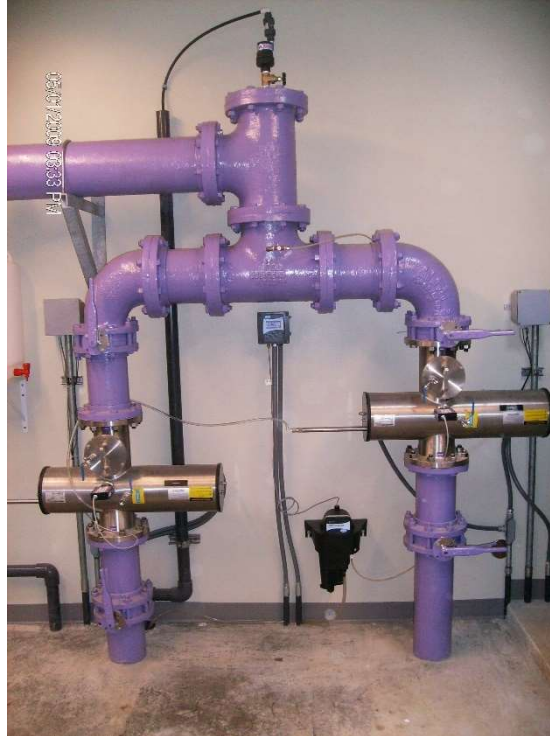
UV Disinfection System
