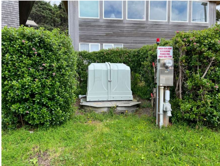
North Pump Station
