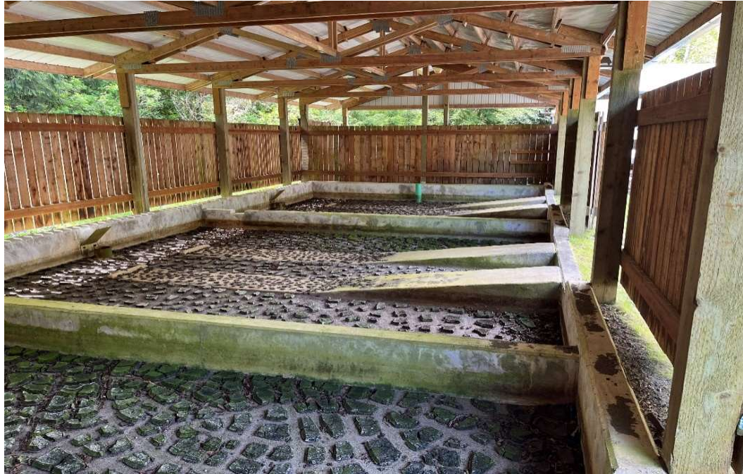
Sludge Drying Beds
