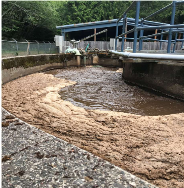
Aerobic Digester No. 1
