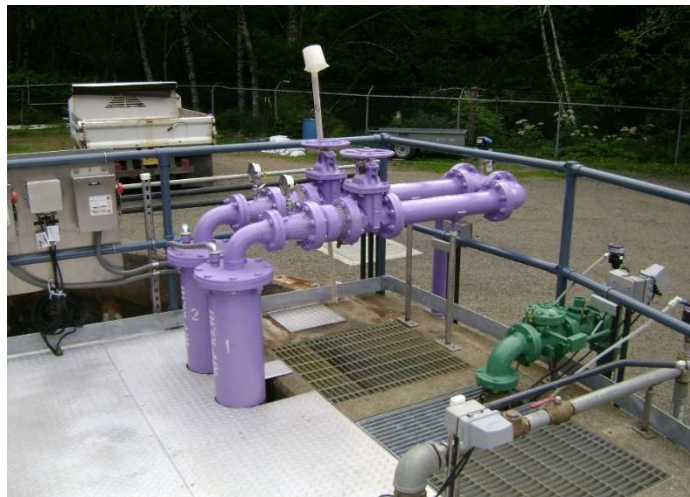
Reclaimed Water Pump Station
