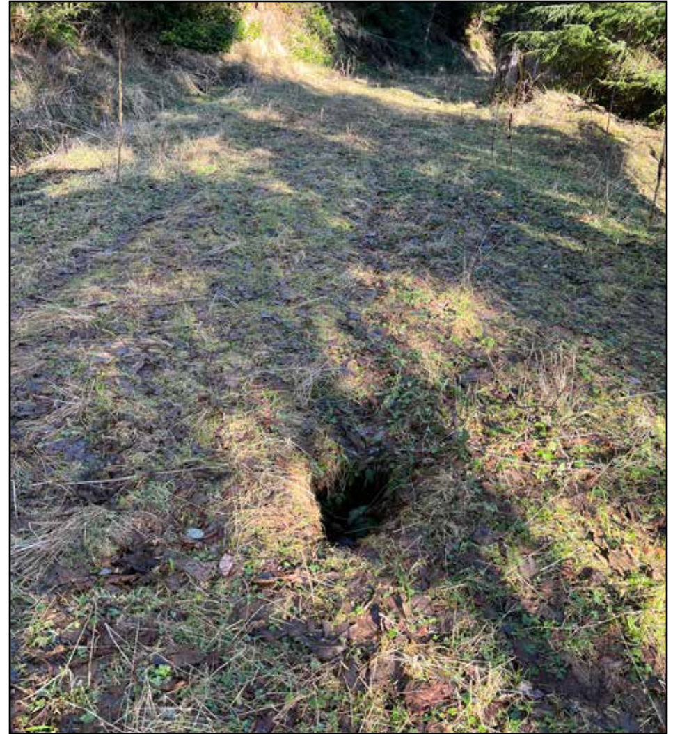
A failing log puncheon creating a hole in the road surface on the Onion Peak Rd. These holes are often very deep and indicate a hollow area under the road.
